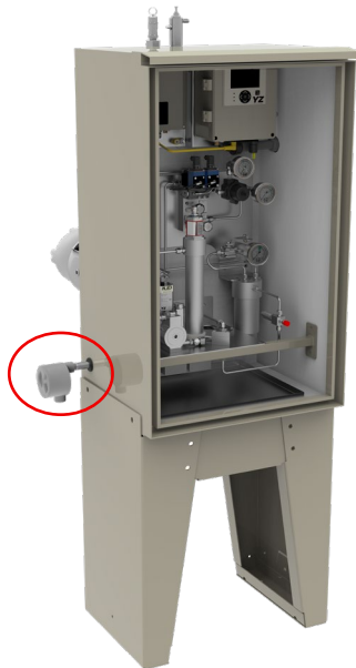
Figure 5 Heater Junction Box Location
