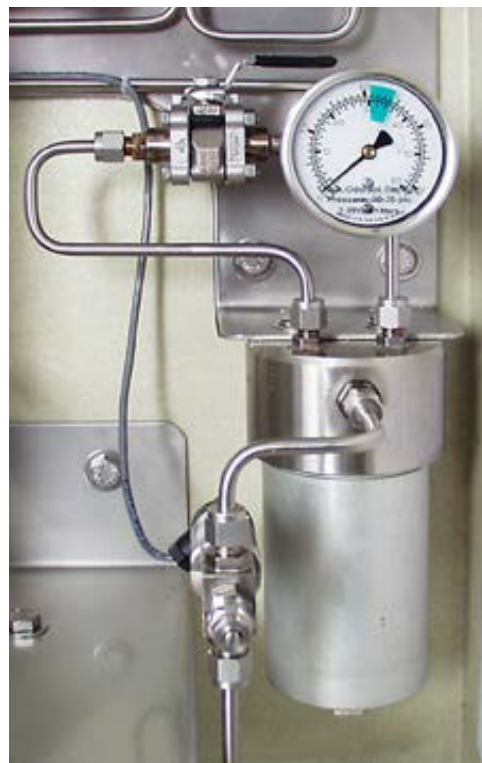
Figure 66 Inlet Manifold, Bulk Odorant Filter
