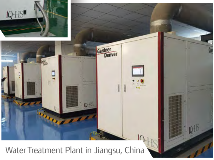
Water Treatment Plant in Jiangsu, China
