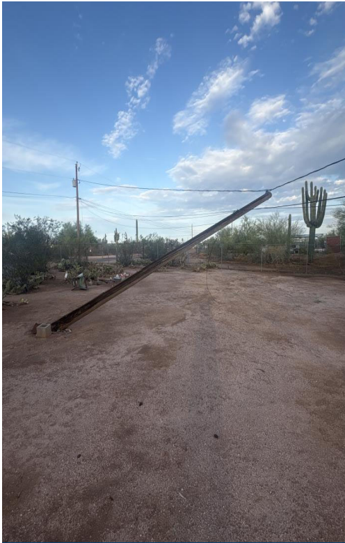
Broken 12kV Pole
