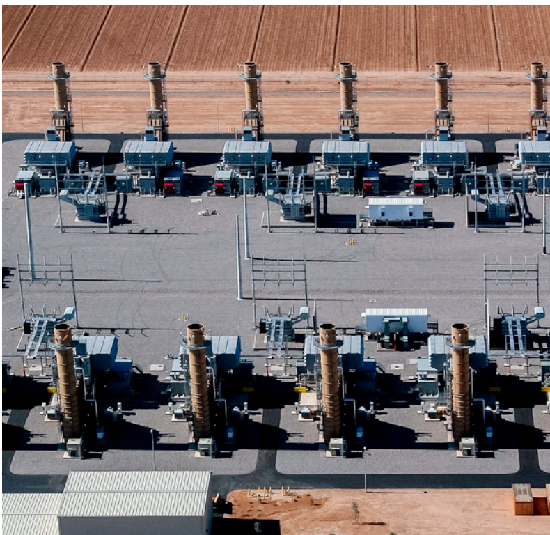
Figure 2: Existing generation units
