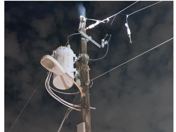
Failed Arrester – Lightning Strike
