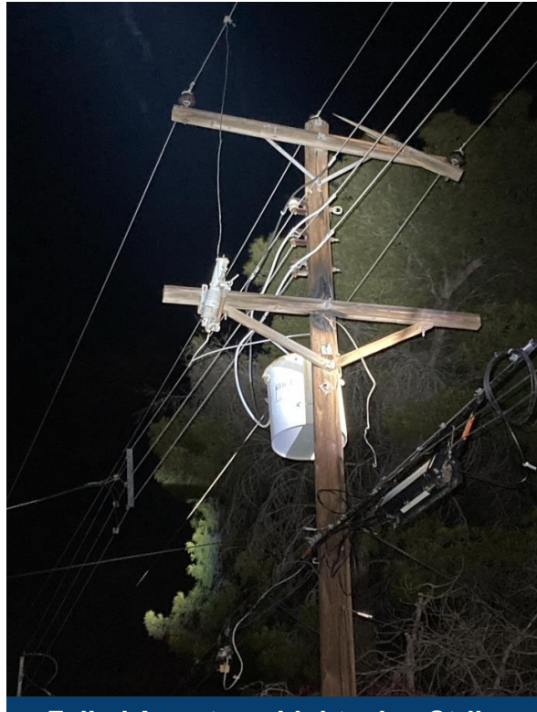
Failed Arrester – Lightning Strike
